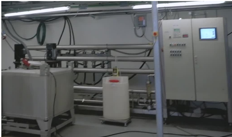
Demonstration scale Nano filtration plant (100 m 2 )
