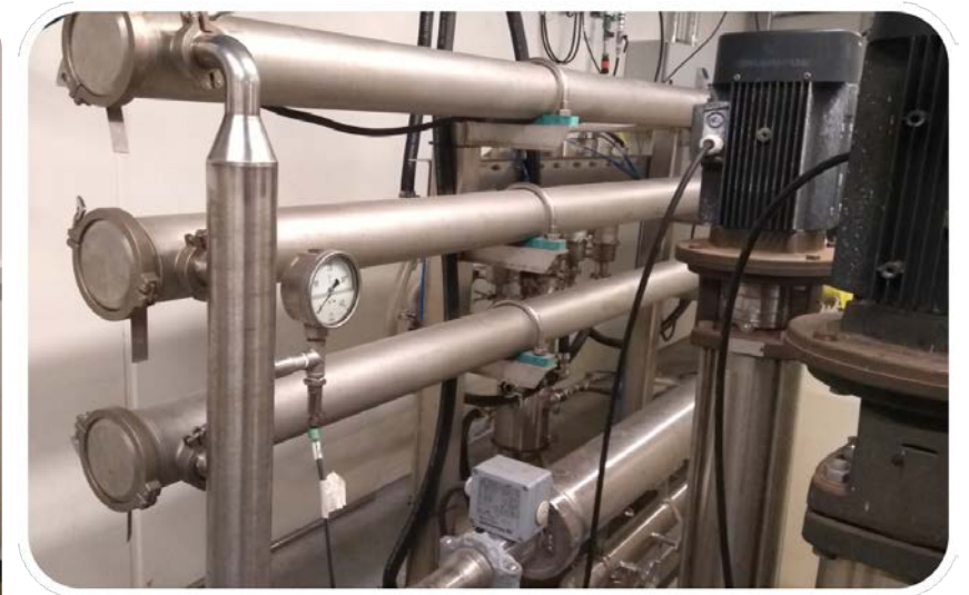
Pilot membrane filtration unit
